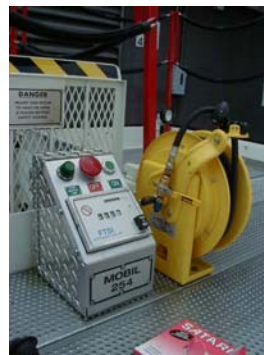
Floor mounted meter and control panel
